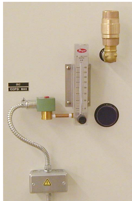
GN2 Purge System
